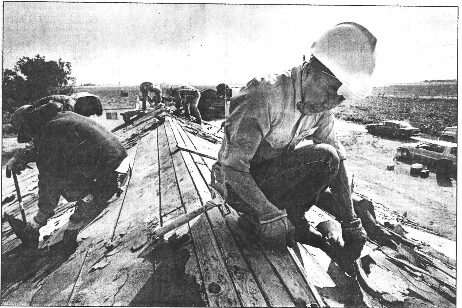
In Wyoming: Volunteers (above and at right below) disassemble the barracks at what was the Heart Mountain Relocation Center during World War II. More than 120,000 Japanese-Americans were incarcerated in the camps during the war years.
