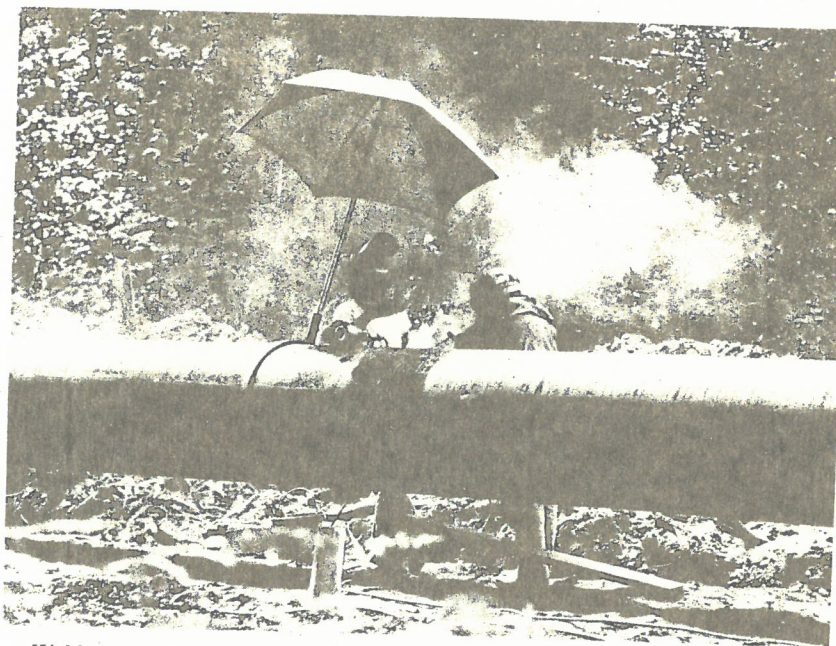
Welders in rainy Washington put final touches on El Paso's Canada pipeline
